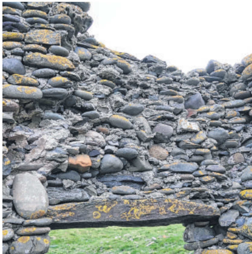
Above a doorway in a shore-stone building – the outer 'slate' lintel survives, but the inner wooden one has failed and the inner leaf of shorestones has fallen to the ground
