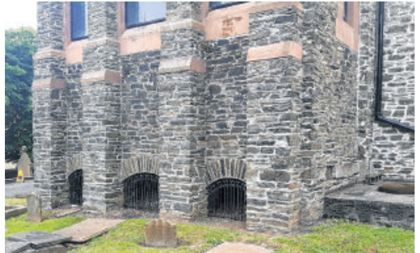
The Apse at St George's supported on piers to avoid disturbing burials beneath
