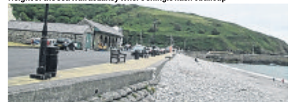
Other parts of the Laxey wall are increasingly ineffective because of the build-up of shingle
