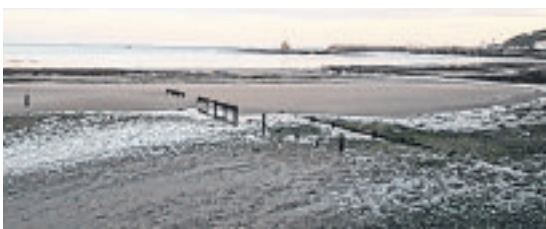
Ineffectual skeletal remains of neglected groyne on Douglas beach, which were recently removed
