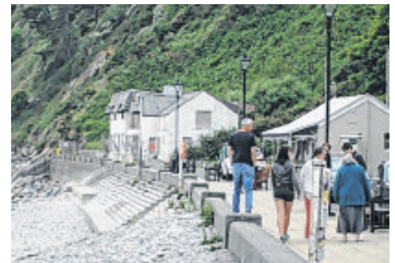
Height of the sea wall at Laxey where shingle hasn't built up
