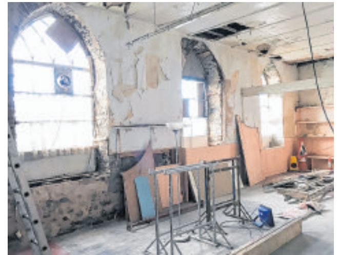
The current internal state of Kirk Michael Courthouse (Chrystals Estate Agents)
